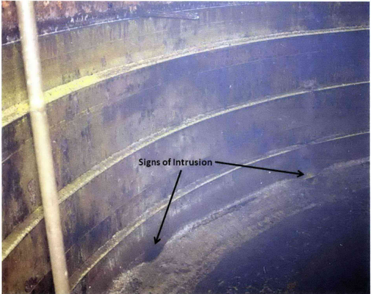
Figure 3-4: Signs of Liquid Intrusion (Tank 241-T-102) 3
