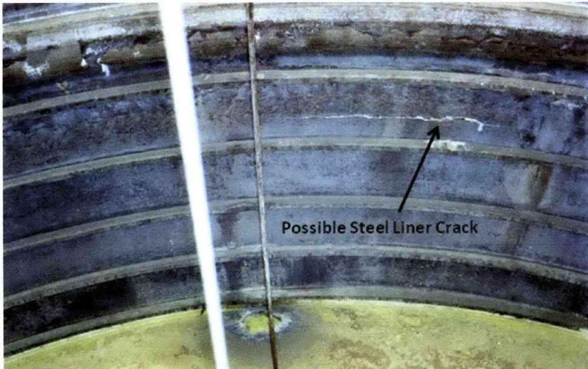
Figure 3-5: Possible Steel Liner Crack (Tank 241-SX-112) 4
