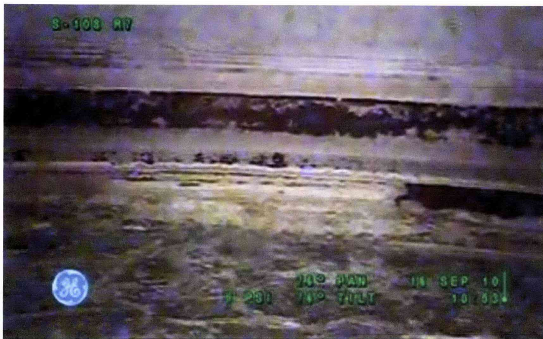
Figure 14-5: Tank 241-S-108 Steel Liner
