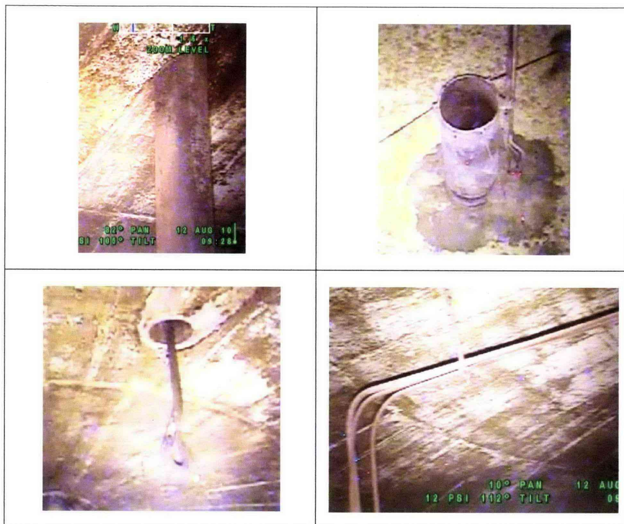
Figure 6-5: Tank 241-A-106 In-Tank Equipment/Risers
