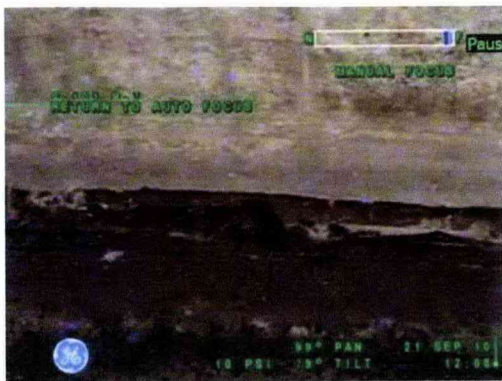
Figure 11-4: Tank 241-S-101 Steel Liner
