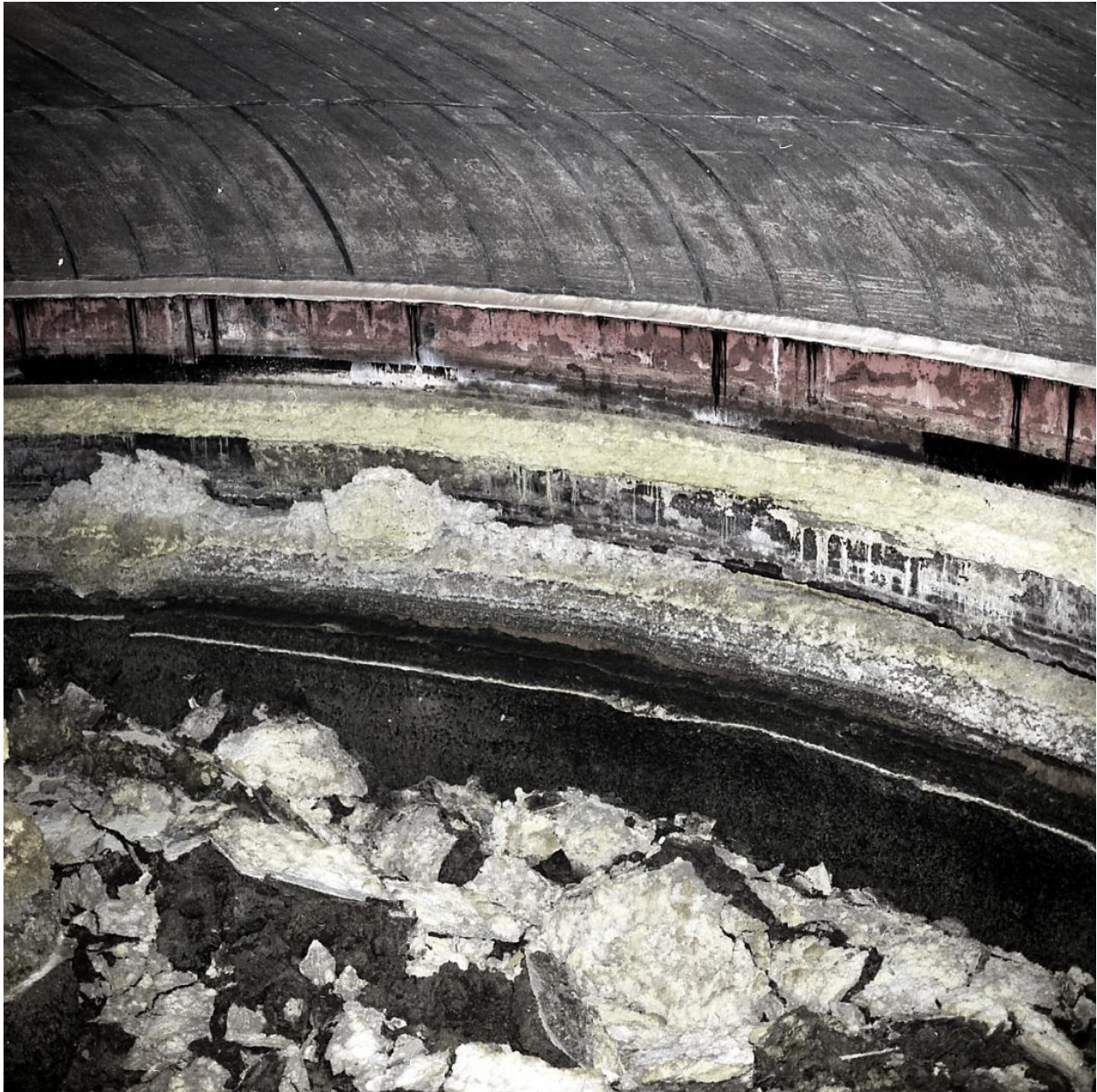
Figure 4-6. Tar Rings Photos for Tank 241-BY-108
