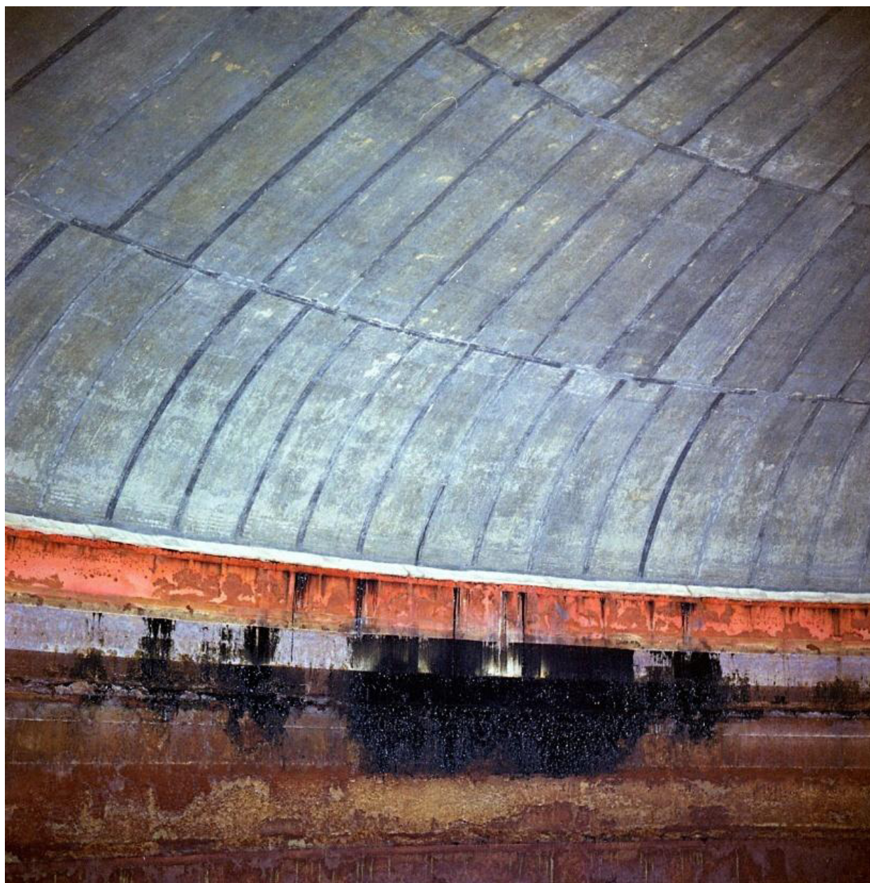
Figure 4-7. Tar Ring Photos for Tank 241-BY-110
