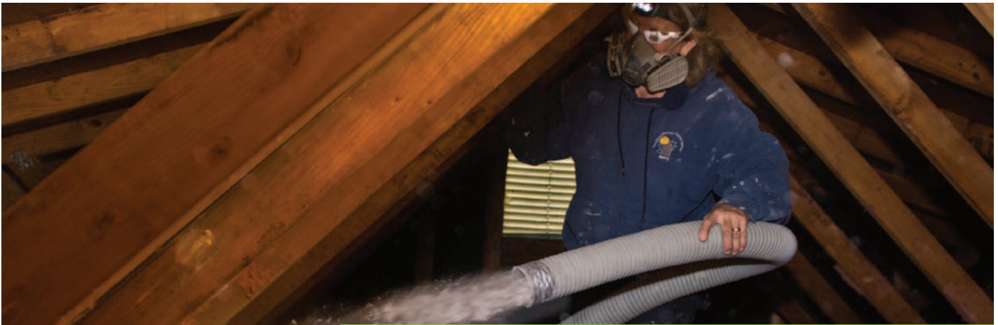
A Weatherization crew member blasts dense pack insulation into the attic and wall cavities of a client's home
