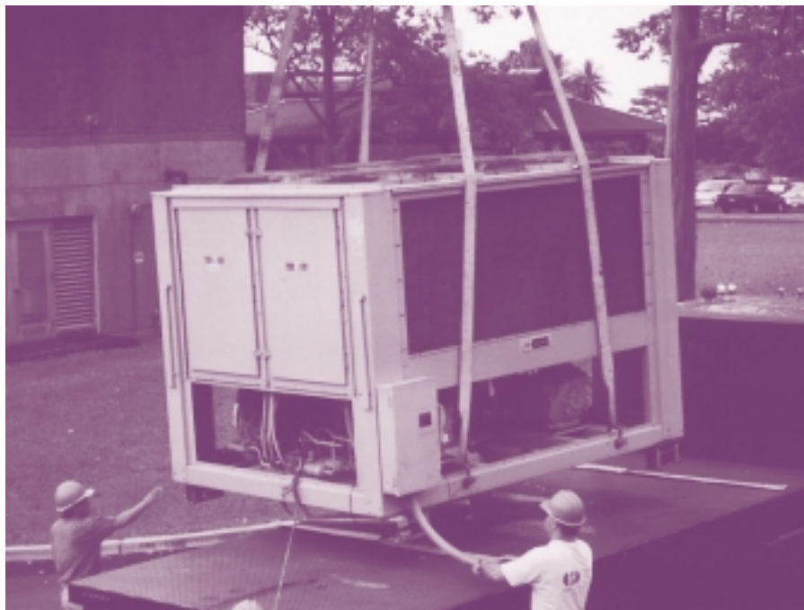
THE REBUILD HAWAII PROJECT PROVIDED FOR THE INSTALLATION OF A 400-TON VARIABLE SPEED CENTRIFUGAL CHILLER AT THE UNIVERSITY OF HAWAII.
