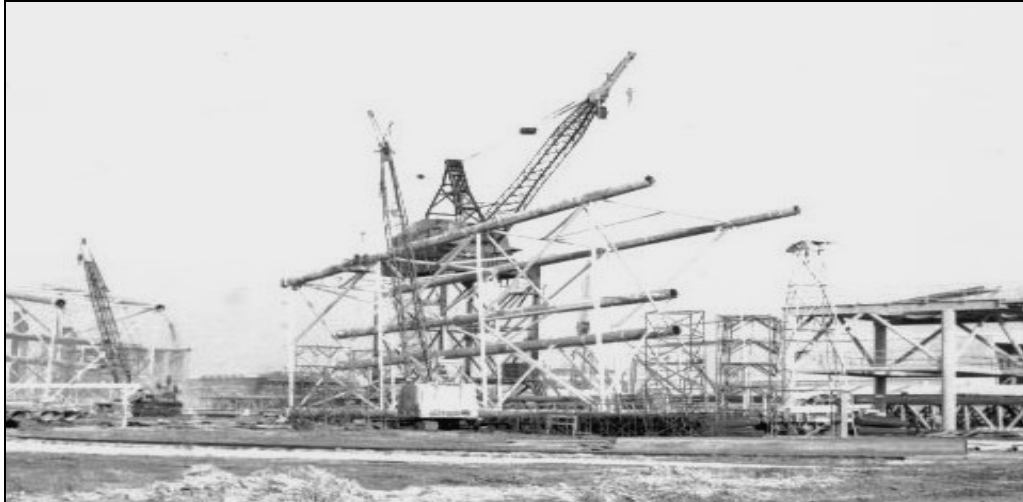
Figure 5.10. Platform under Construction at McDermott Yard in Amelia. Photo Courtesy of Dolores Henderson, OOGHP.
