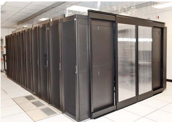
Figure 23. PPPL's hot aisle containment enclosure. Photo courtesy of PPPL
