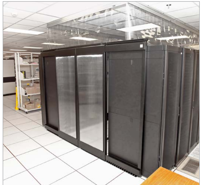
Figure 12. PPPL's computing environment. Photo courtesy of PPPL.
