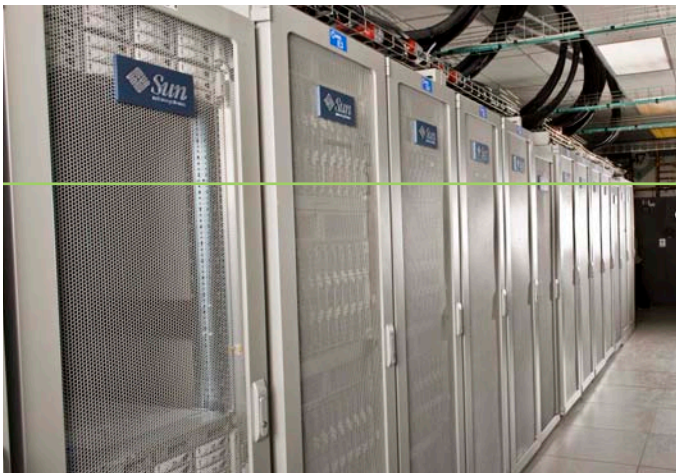
Figure 42. Sandia’s Red Sky HPC. Photo courtesy of Sandia National Laboratories
