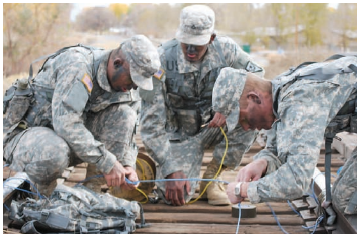
From left, Privates First Class Randy Jackson, Craig Kenison and Adam Brayton set up their explosives at one end of the Coleman Road Bridge during a training exercise in Fallon in November.
