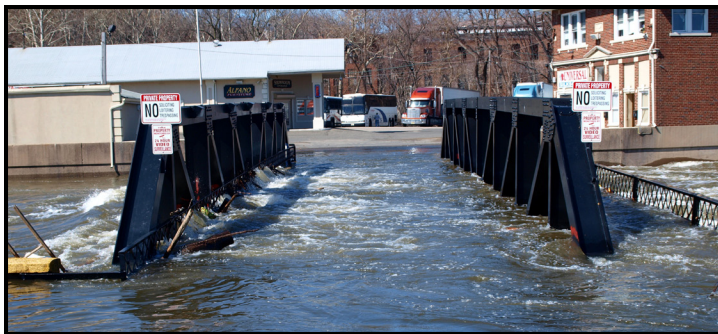
Alfano Island Bridge over the Passaic River (Photo courtesy of Mario Burger)
