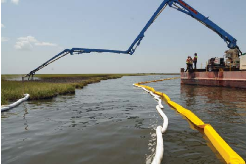
HOPEDALE, La. – A concrete pumper has been converted into a shallow water skimmer and marsh washing system used to remove oil from the shoreline. Photo courtesy of U.S. Coast Guard
