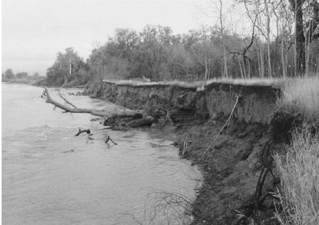
Figure 2.8. Active bank erosion illustrated by vertical cut banks, slump blocks, and falling vegetation.
