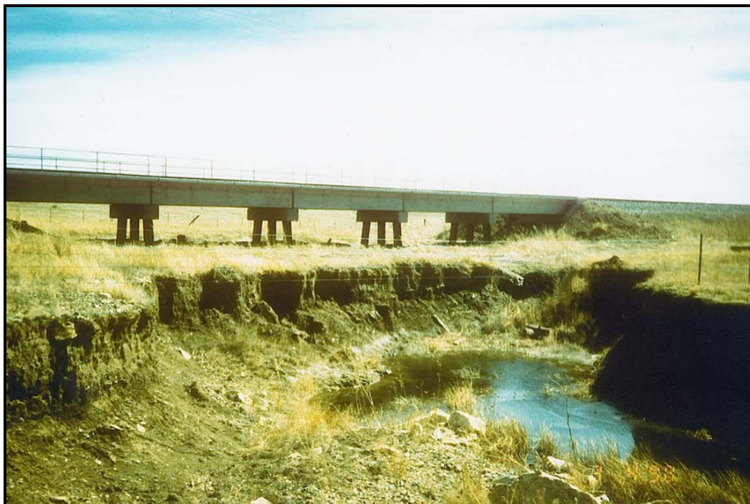
Figure 6.18. Headcut downstream of bridge.
