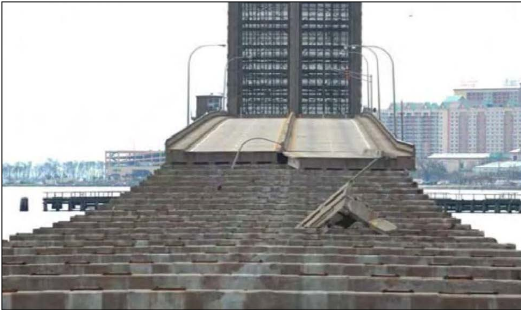
Figure 10.6. Photograph of a bridge damaged by Hurricane Katrina from HEC-25 (FHWA 2008).
