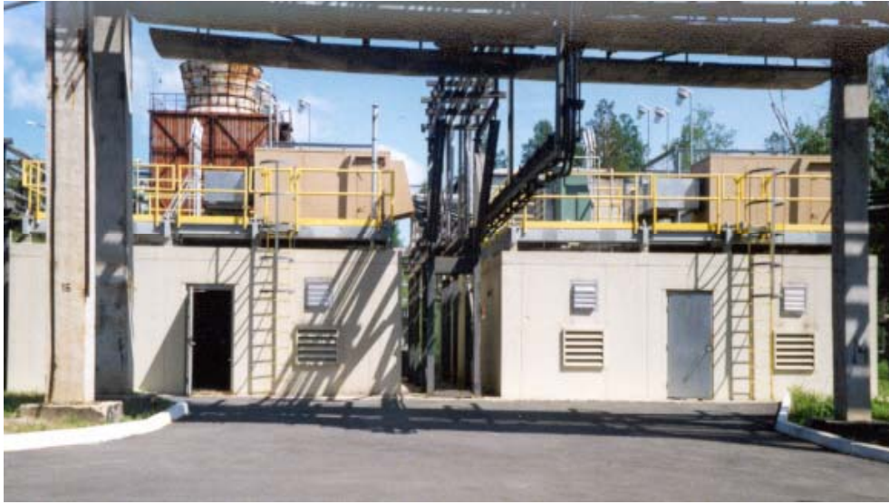
Figure D-5. Hydrogen Generator Buildings (One for Each Disposition Unit)
