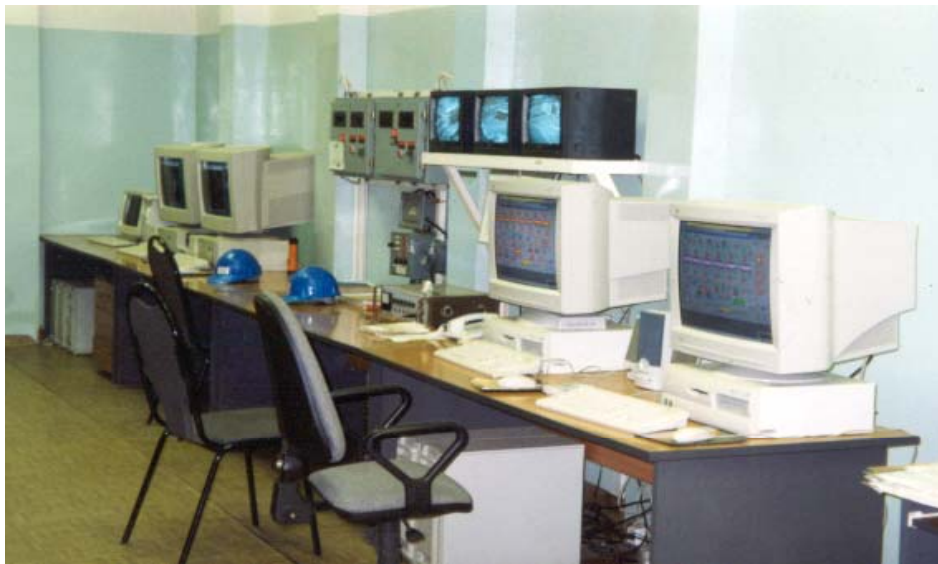
Figure D-8. Interior of the Computer Process Control Room
