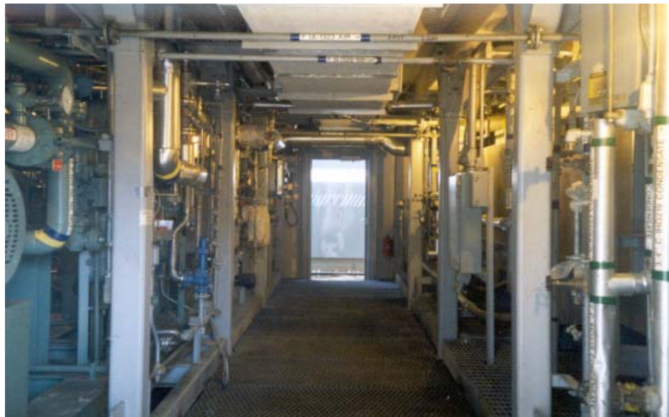
Figure D-4. Interior of One of the Two Heptyl Disposition Units
