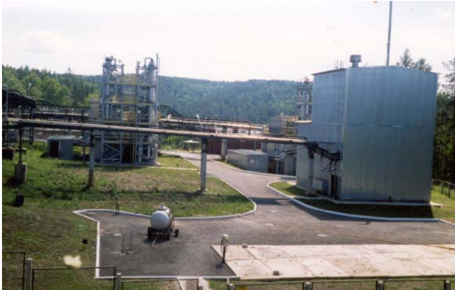
Figure D-2. Ground View of the Heptyl Fuel Disposition System
