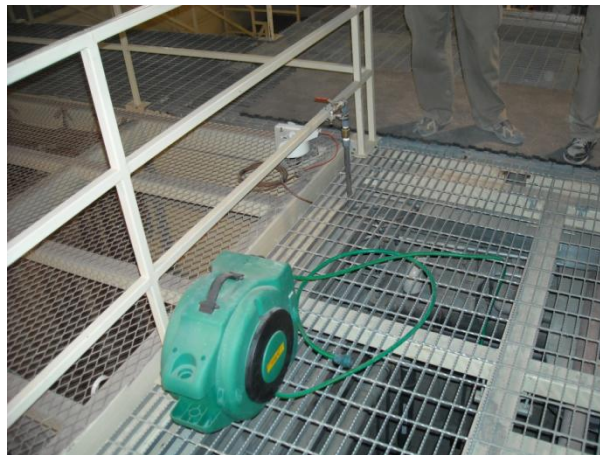
Figure 8. Interim Fix to Fire Suppression System
