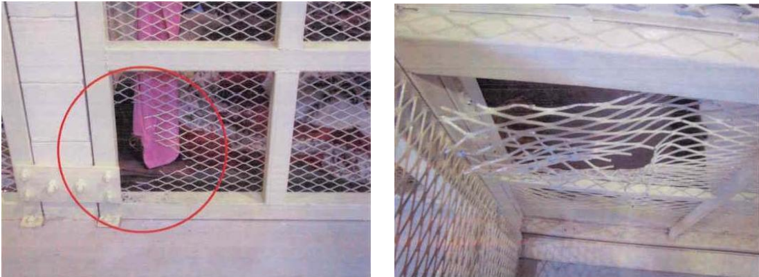
Figure 2. Examples of Cell Damage
