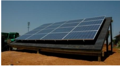
The Clean Energy Technology Training program includes hands-on training with clean energy equipment.
