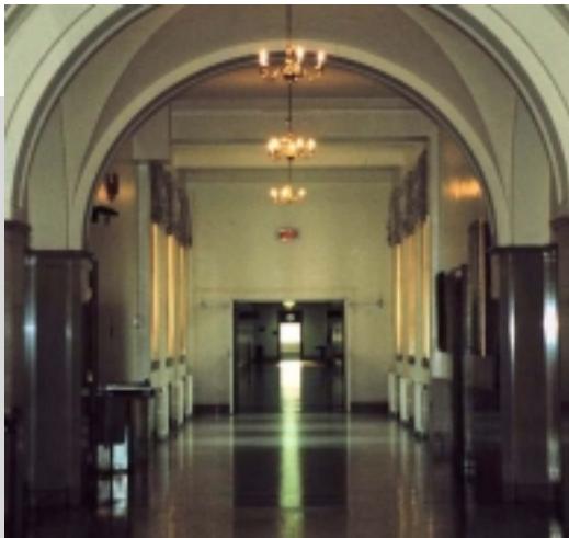
Fig. 11: Standard drywall partition with 90 minute rated doors for cross corridor fire separation reduces height and width clearance. New products offer alternatives that maintain corridor clearance.
