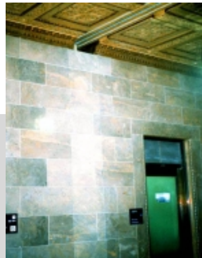
Fig. 16: Accordion door tracks, receiving slot and cover painted to match marble walls and coffered ceiling. Commerce Dept, Washington, DC.
