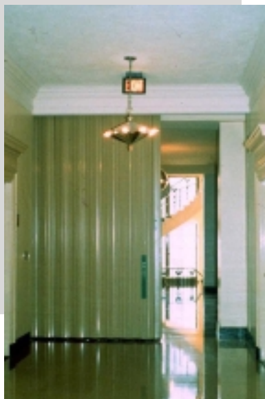
Fig. 15: Bulkhead installed below vaulted ceiling to accommodate track for WON door. If space above ceiling allows, entire door can be retracted to maintain vaulted ceiling clearance. Ariel Rios building, Washington, DC.
