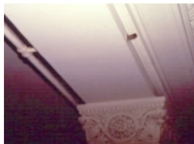
Fig. 8: Detail showing exposed pipe tucked behind beam. Old Post Office, Washington, DC.
