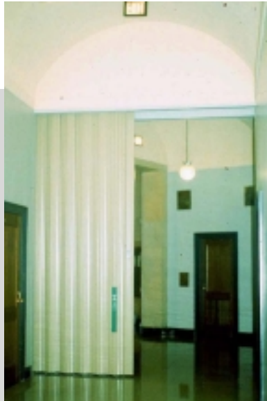
Fig. 14: WON door accordion fire partition (partially retracted) allows ceiling and wall clearance to be maintained. Ariel Rios building, Washington, DC.
