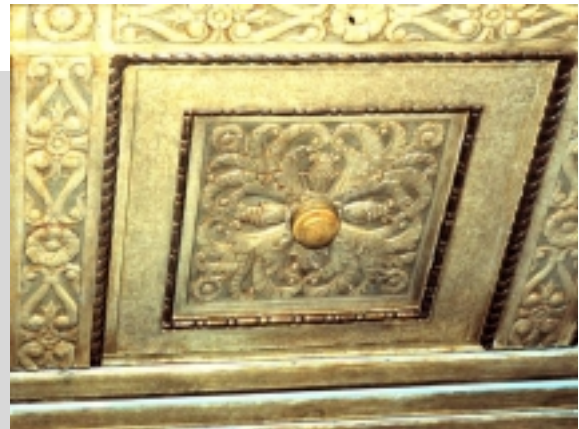
Fig. 5: Recessed smoke detector in ornamental plaster ceiling at the Commerce Dept., Washington, DC. All surfaces but the detector head were painted to match the ceiling.
