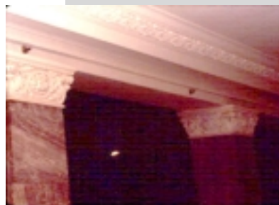
Fig. 9: Only the sprinkler heads are visible from principle vantage points within the corridor.
