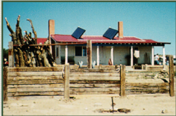
Solar installation at Pueblo of Laguna's Majors Ranch
