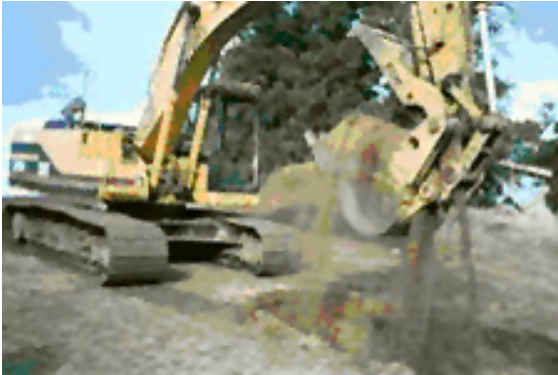
The Rio Vista, Calif., U.S. Army Reserve Center was the first site to use GFPR to complete regulatory closure.
