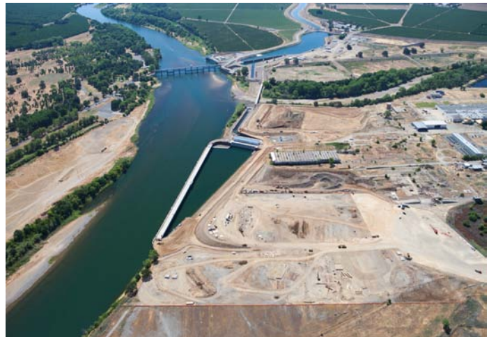
Red Bluff Pumping Plant and Fish Screen.
