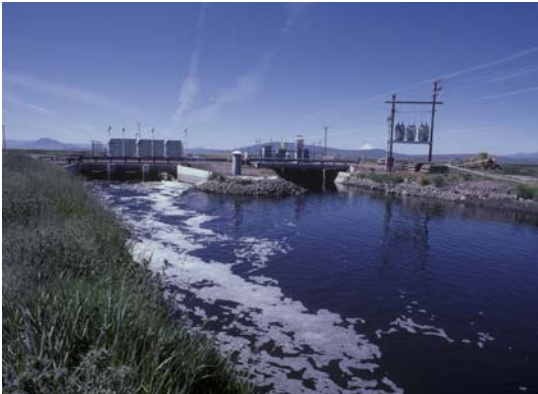
Pumping plant E and EE on the Klamath Straits Drain.
