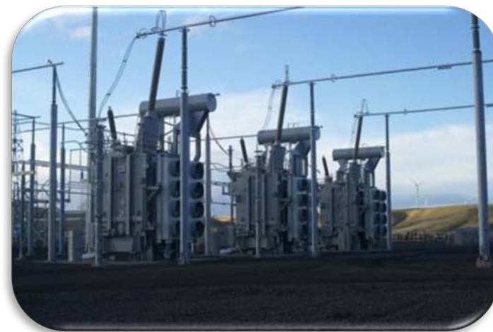
Central Ferry Substation
