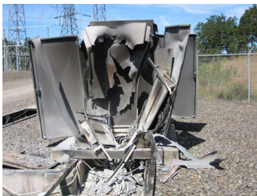
Figure A-1.1 Collateral Damage from Attempted Metals Theft
