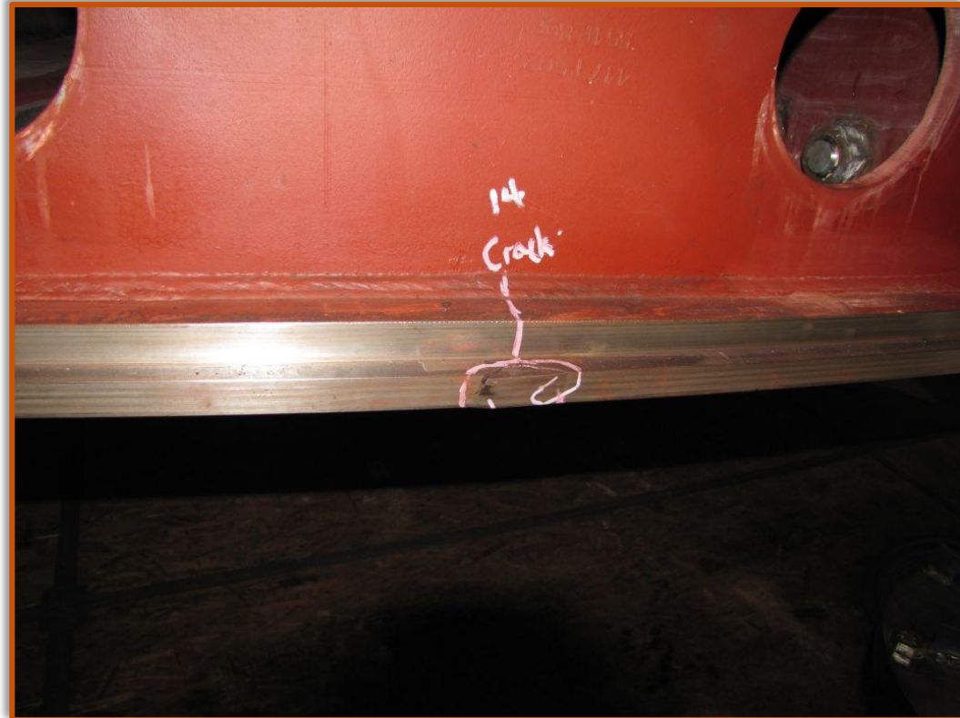
Crack in bottom of spider where it fits to the rim
