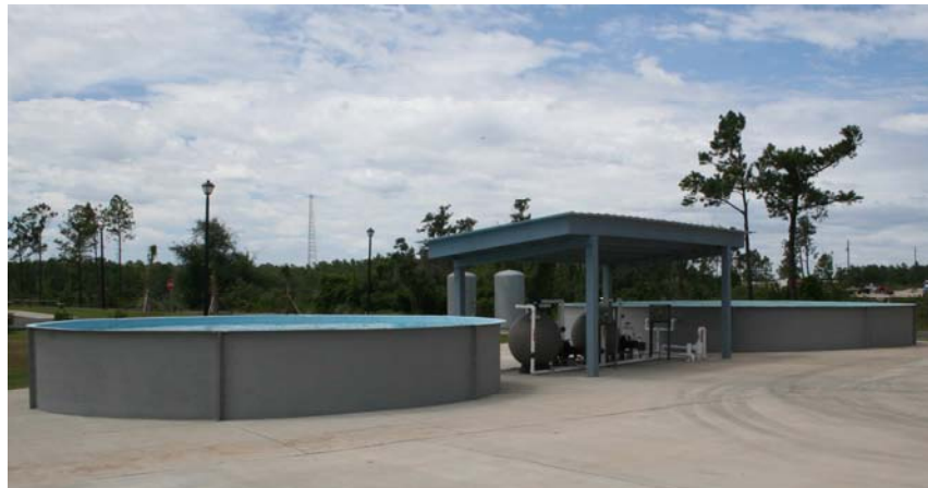
Water treatment and mixing pools for rehab area with wells in background (west of animal care building).
