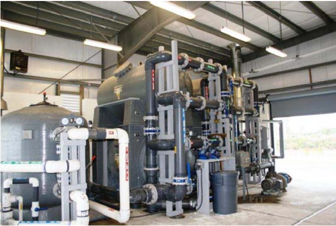
Life support systems (pumps and filters) in Animal Care building.
