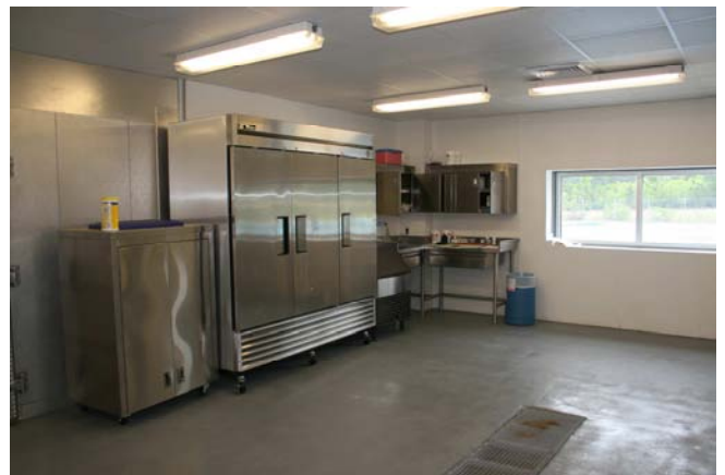
Another view of the fish kitchen with refrigerator and stainless steel cabinets and counter (view of pools through window).
