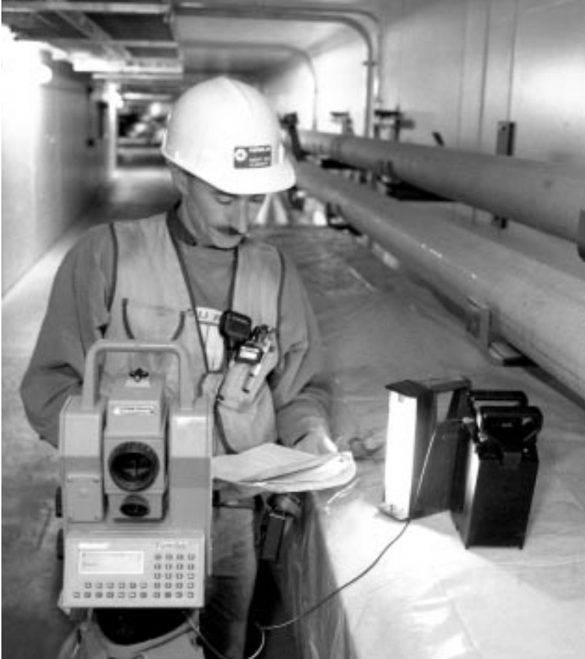
Gary Coppola uses a geodimeter to check angles during construction of the Main Injector.
