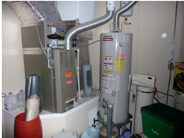
Figure 53. A gas furnace is located on a support platform used as the return plenum located inside a garage next to a gas water heater. Return leakage can depressurize the garage and interfere with proper venting of these atmospherically vented gas appliances.
