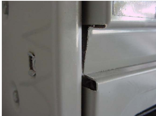
Figure 46. Close-up view of lower corner AHU panel leakage.
