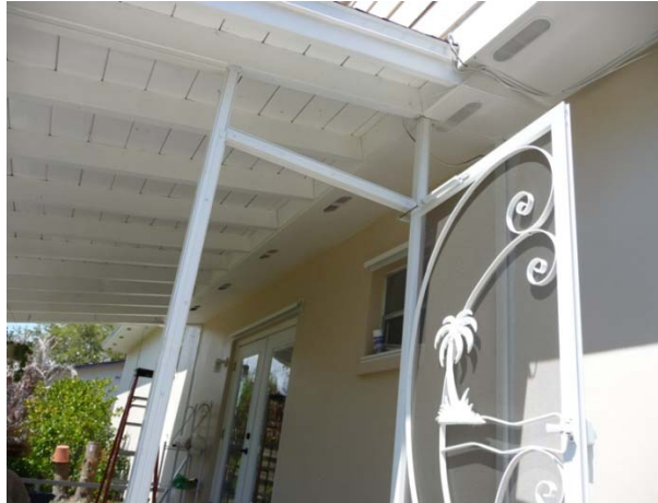
Figure 35. Oval shaped soffit vents can be seen on the underside of cantilevered floor section.
