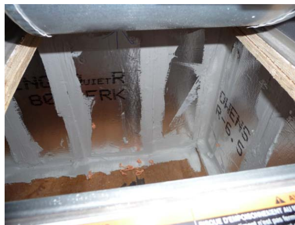
Figure 57. View inside a support platform sealed using ductboard with foil (which is the air barrier) facing inward so seams can be sealed at the foil air barrier with mastic.
