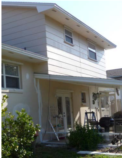
Figure 34. Second-story floor cavity has cantilevered section that was vented on the back side of home.
