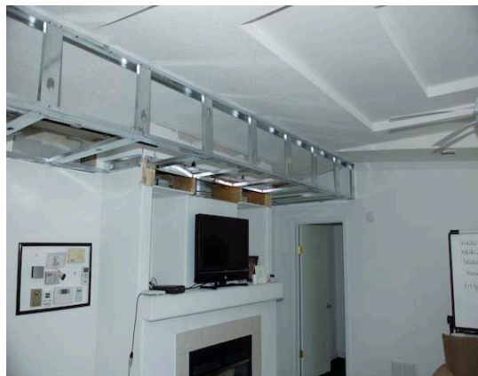
Figure 15. Interior duct system under construction. Metal framing is used to construct a chase that will hide the ducts from view once covered with drywall. The chase should be tight to the attic and leakier to the room.
