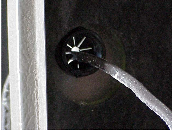
Figure 48. Leaky thermostat wire penetration.
