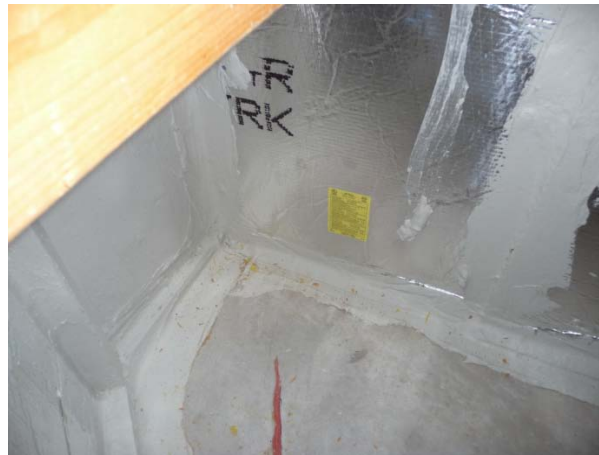
Figure 59. All seams in this support platform return plenum have been sealed using mastic.
