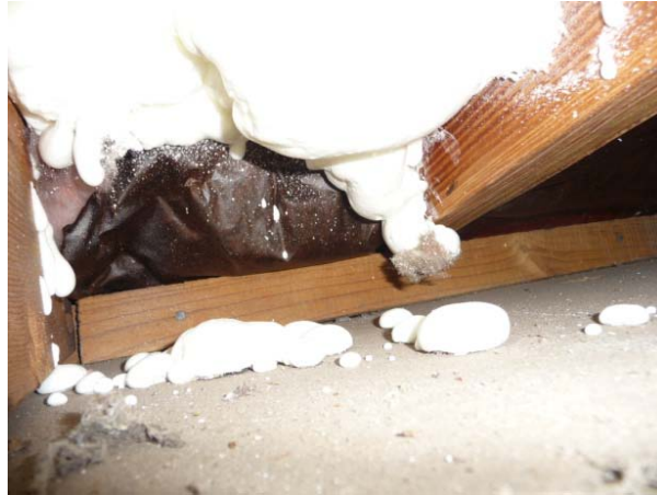
Figure 38. First, the foam spray gun is inserted into the soffit vent hole to apply foam insulation to the floor deck above, beyond the top of the exterior wall.
