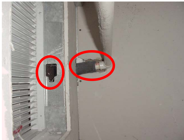
Figure 62. Grille transfer through a wall has leakage into wall cavities that need to be sealed.
