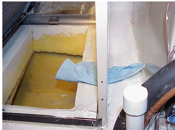
Figure 51. Blue cloth has been pulled under AHU cabinet to illustrate air pathway where the return plenum and the AHU join together.
