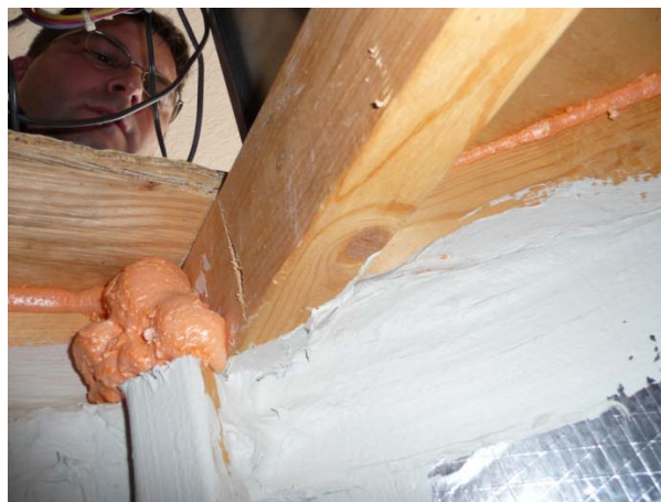
Figure 60. All penetrations and junctions between duct board, structural, and panel components of the return plenum have been sealed.
