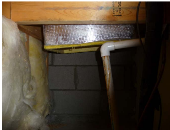
Figure 56. View inside a return plenum located in a garage. Air leaks are drawn primarily from the garage, but a small portion comes from the attic down through the wall cavity where the insulation is located. The block wall in the background is an exterior wall.
