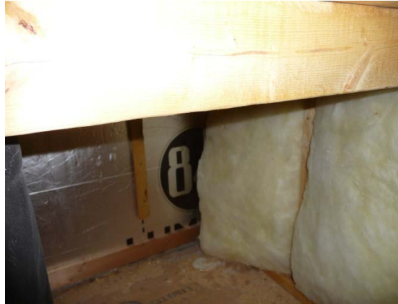
Figure 55. View inside a return plenum located in a second floor closet shows lack of effective duct air or thermal barrier. Attic air could be drawn down leaks in wall cavities and through the floor cavity, which is also well connected to an attic space.
