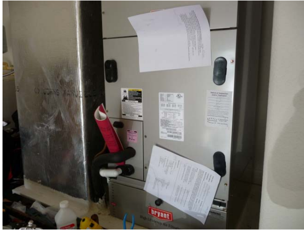
Figure 45. AHU panel leaks are strong enough to hold sheets of paper.
