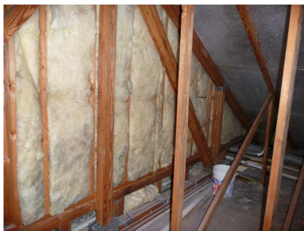
Figure 21. View of kneewall and portions of open floor cavity as seen from inside the garage attic.
