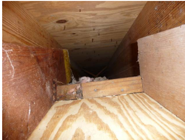
Figure 36. Connection from vented eave to floor cavity where no insulation was found.
