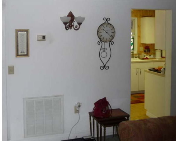
Figure 61. The interior of a return plenum, located under an AHU, can be accessed through the return grille for inspection.
