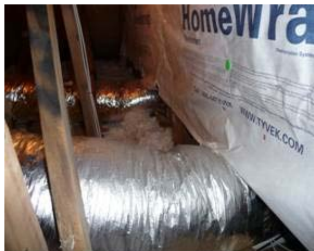
Figure 11. Flex ducts going from an attic space into the interstitial floor cavity under a portion of the second story conditioned space.
