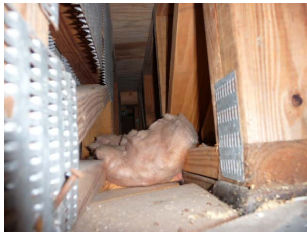
Figure 29. View from the vented eave cavity that is well-connected to second-story floor cavity.
