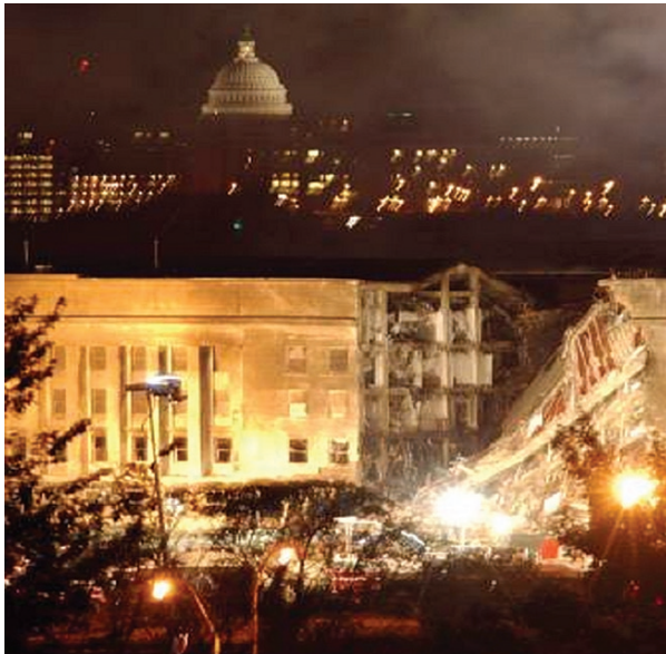
Rescue crew and fire fighters work through the night
