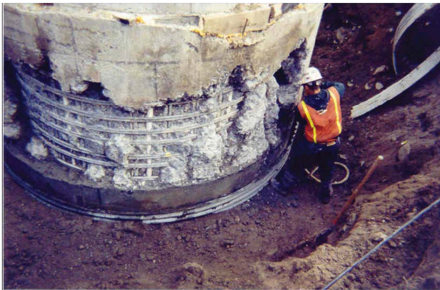
Figure 6: Drilled shaft with defects due to loss of workability
