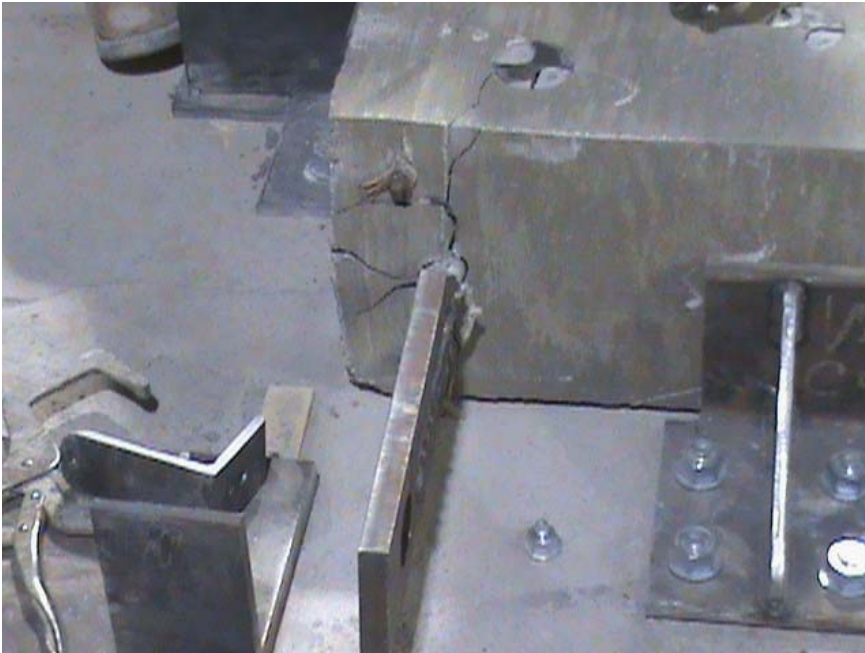
Figure 48: Typical pullout failure.
