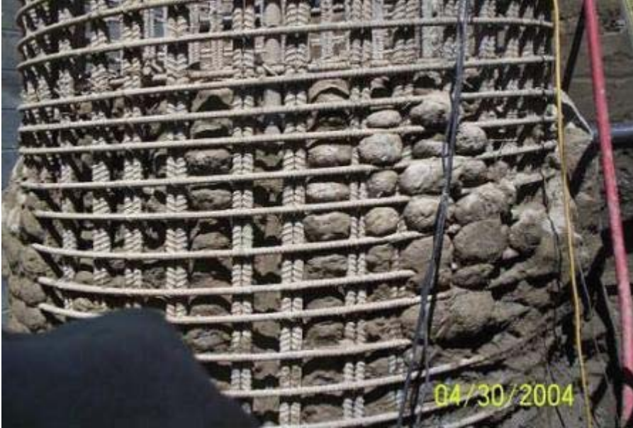
Figure 5: Drilled shaft not encapsulated by concrete [19]
