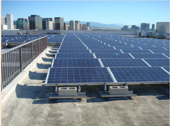
Solar Photovoltaic System at the West Los Angeles VA Medical Center.
