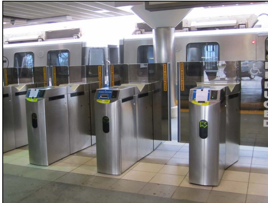
Figure 15: Passenger Access Control Gates at a Subway 26
