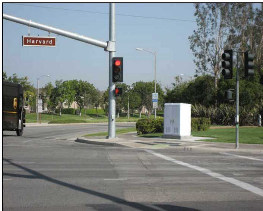
Figure 6: Traffic Signal Control Box 14
