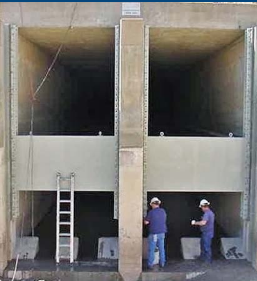
Installing flow deflectors at Choke Canyon Dam is just one way Reclamation’s Research and Development Program has put basic research into action. See the featured patent on page 13.
