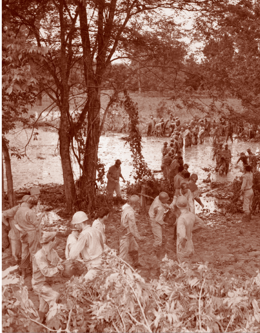
Soldiers of the 359th Engineer General Service Regiment repaired a slough in the Jackson Bayou levee along the White River during the 1943 flood. Troops on the far bank filled sandbags, which were handed over the water for placement on the near side.
