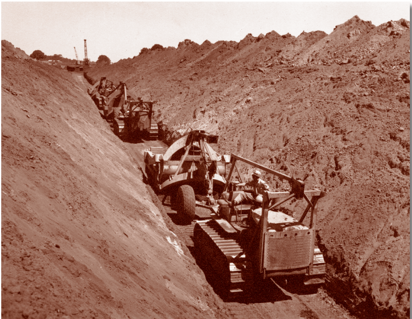
Engineers used heavy equipment to excavate Snead's Canal near Marianna, Florida, June 1948. The deepened canal drained floodwaters away from roads and buildings.
