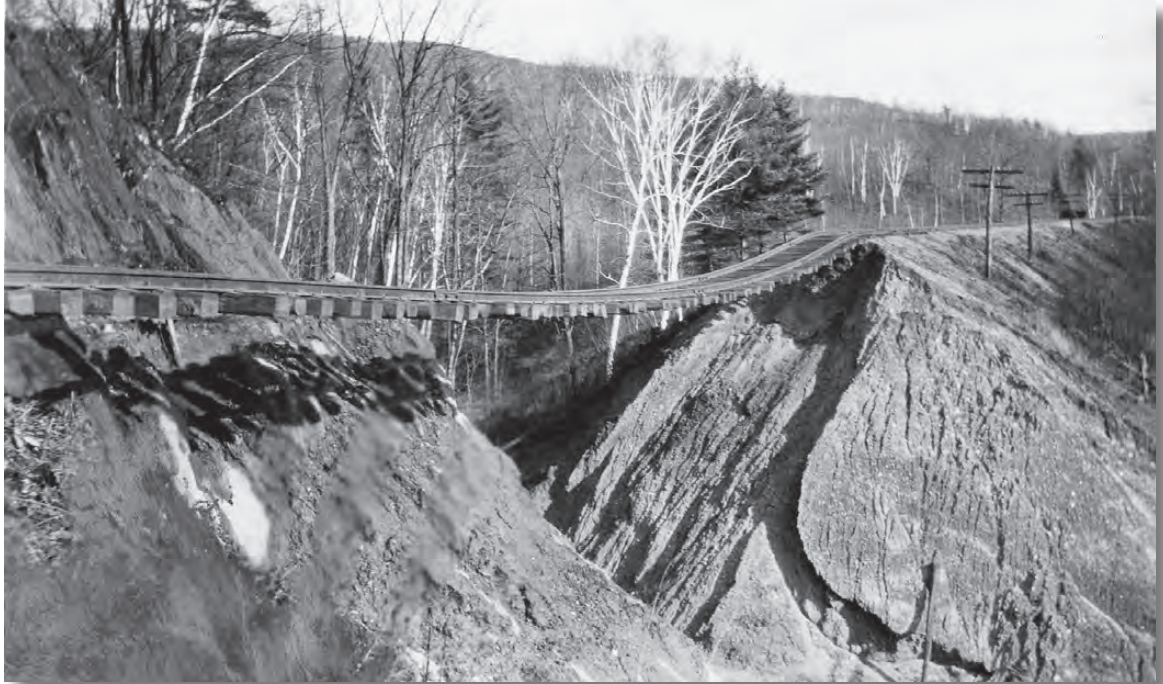
Caving banks undermined a railroad in Vermont, 1927.
