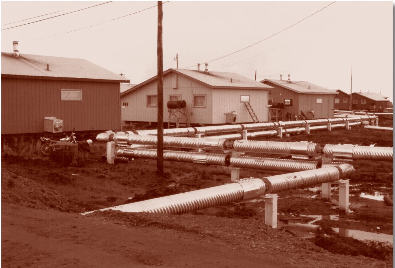
A fire in remote Bethel, Alaska, in 1978 left the town without water and sewer service. The Corps of Engineers designed and built an emergency above-ground replacement system so innovative that it won an engineering design award.
