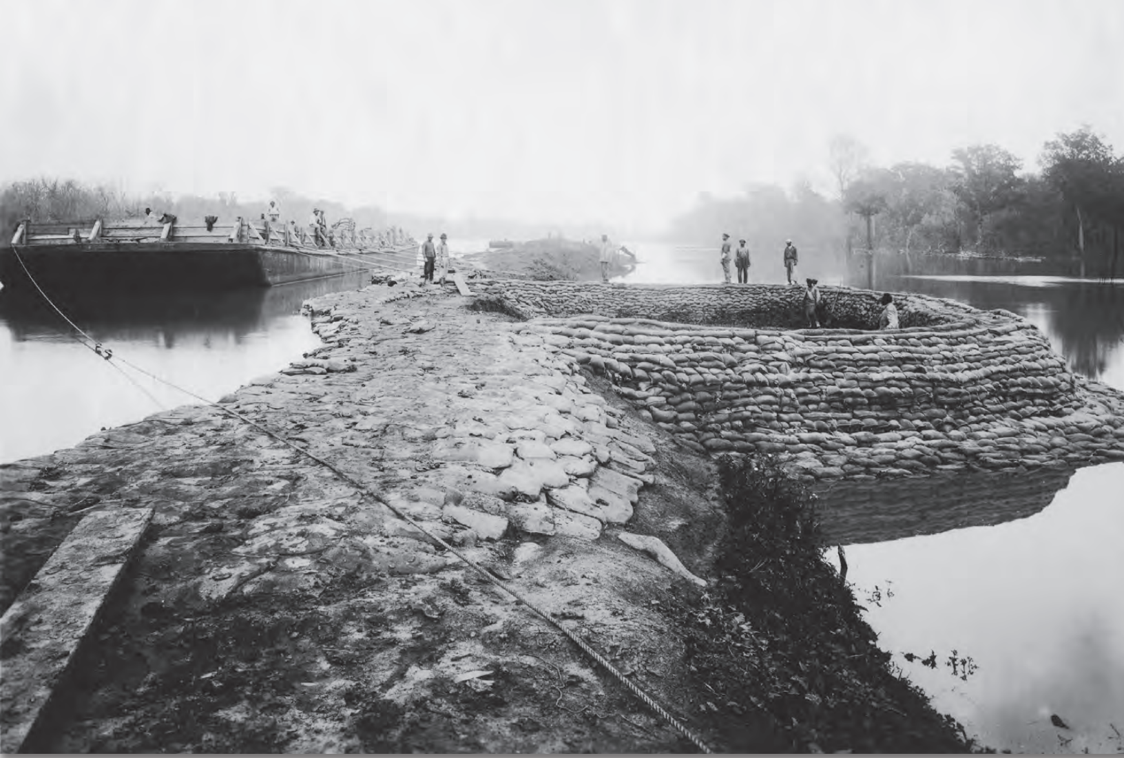
Workers added reinforcements to a threatened break in Ashbrook Dike on the Mississippi, 26 April 1922.
