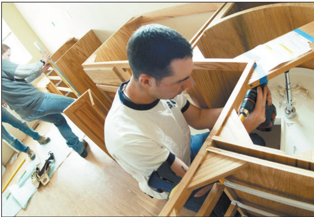
Cadet 1st Class Brian Finneran of CS-08 installs a lazy susan while Cadet 3rd Class Michelle Parenteau of CS-22 (in the background) aligns other kitchen cabinets at a house in Habitat for Humanity's Mesa Vista subdivision project in Montrose, Colo.
