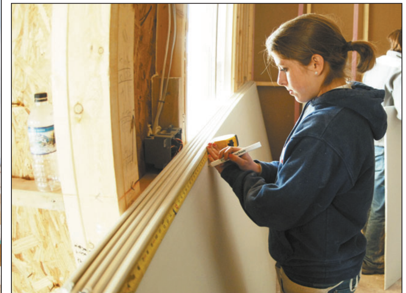
Cadet 4th Class Caitlin Glitz of CS-02 measures drywall for the interior of one of the houses cadets were working on in the Oshara Village project.
