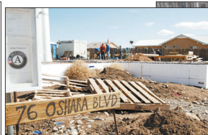
Cadets, right, build pieces of wall frame, for a house that will go up at 76 Oshara Blvd., above, in Habitat for Humanity's Oshara Village project in Santa Fe, N.M.
