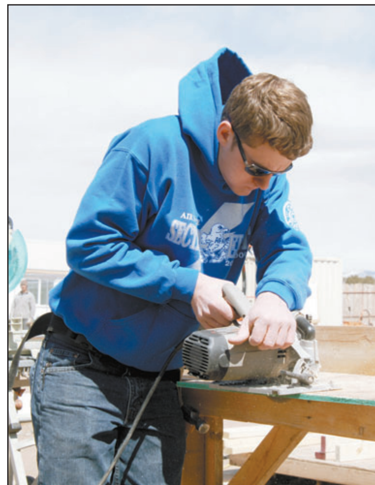
Cadet 2nd Class Billy Baker of CS-40 cuts plywood to be used as part of the wall frame of the house.
