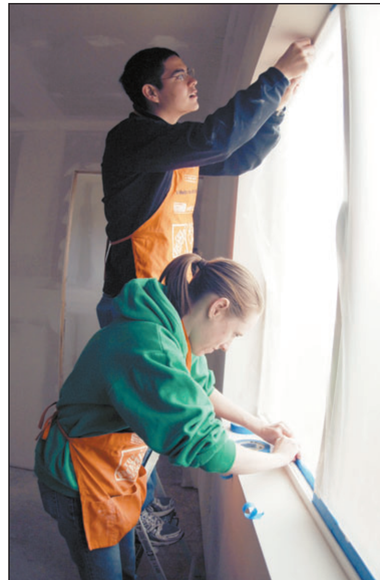
Cadet 2nd Class Chris Horn, top, and Cadet 3rd Class Kristen Lorch tape a window to prepare a room for painting.
