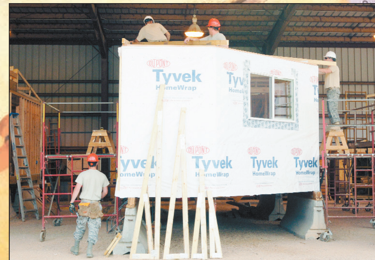
Above: Cadets and CE mentors continue construction on one half of a Navajo Hogan. The Hogans are built in halves to allow transport via an 18-wheeler to the reservation. Right: Cadet 2nd Class Stephen Caple surveys a worksite to determine changes in elevation, during a timed exercise.
