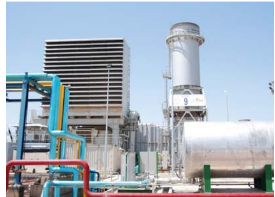
The Qudas power plant, an MOE-run plant on which the United States has spent more than $250 million, had an average output this quarter of 429 MW, which is 47% of its nameplate capacity. (USACE photo)
