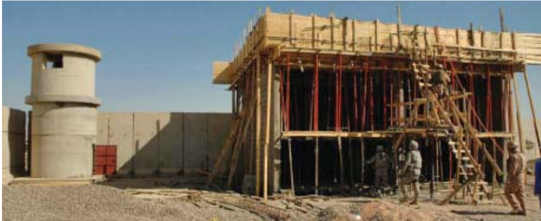
Engineers from GRD inspect the progress of work at the Muhammadi Police Station in Anbar province. (GRD photo)
