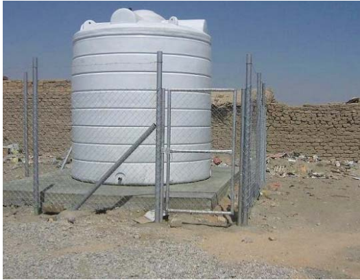
Water tank installed at Al-Zahour, Qadissiya province. (OPA photo)
