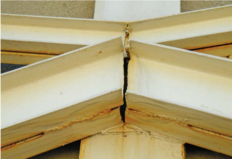
Exterior support damage at the Secure Document Storage Facility.
