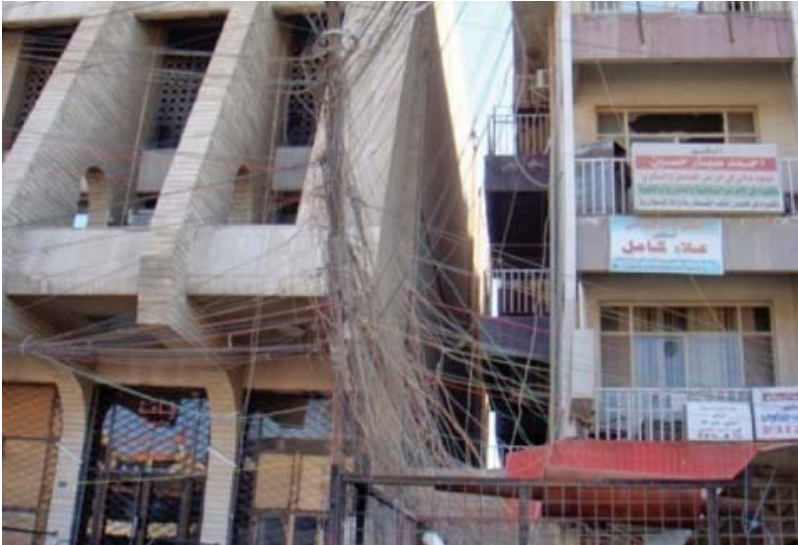
A tangle of consumer-installed electric wires carries power from private generators to at least half the households in Central Baghdad. (Parsons Brinckerhoff photo)
