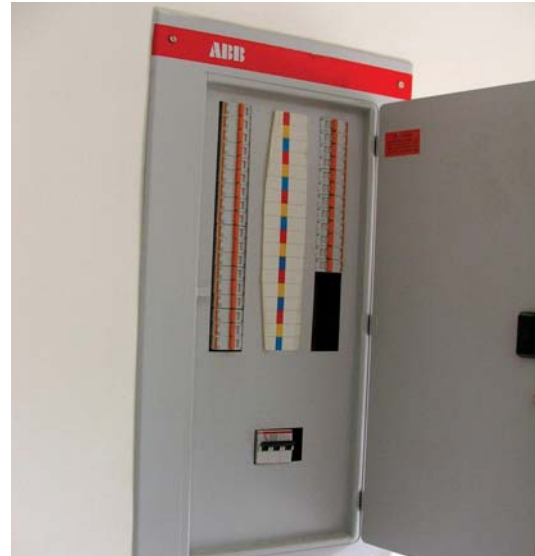
Primary circuit breaker panel with no barrier, Orphanage and Senior Citizen Assisted Living Center.
