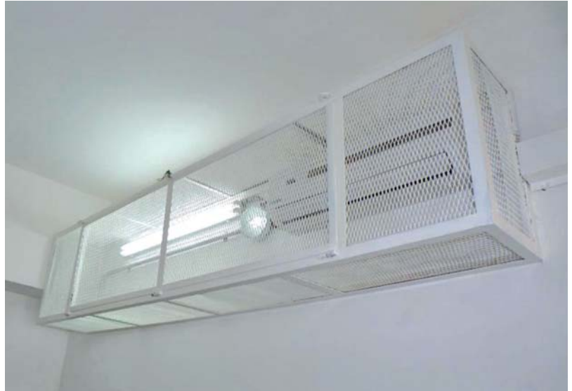
Metal cage protects the HVAC, light, and electrical wiring at Chamchamal.
