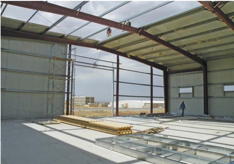
Maintenance garage prior to completion of exterior panel installation at Al Kasik.
