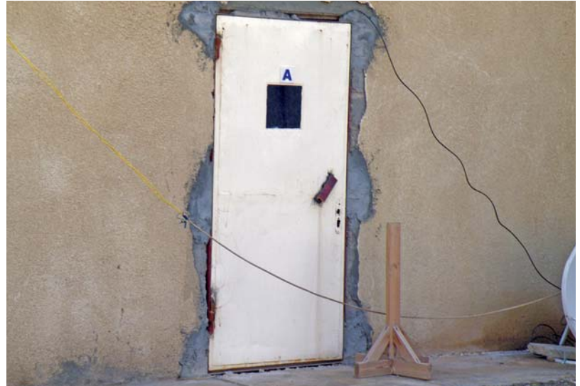
Poorly installed door at the Secure Document Storage Facility.
