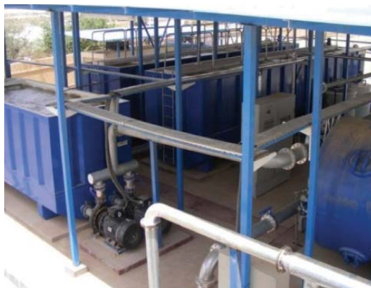
Al-Jihad Water Compact Unit produces 200 cubic meters of water per hour in Wassit province. (OPA photo)
