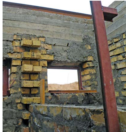
Bond beam increased depth in lieu of lintel in latrine building at Al Kasik.
