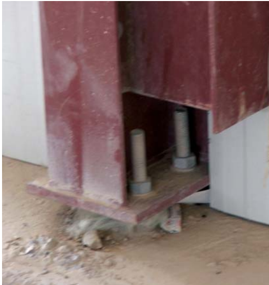
Column base plate prior to placement of non-shrink grout at Al Kasik.
