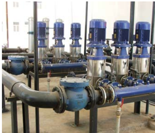
Two sets of booster pumps for circulating potable water throughout the garrison
