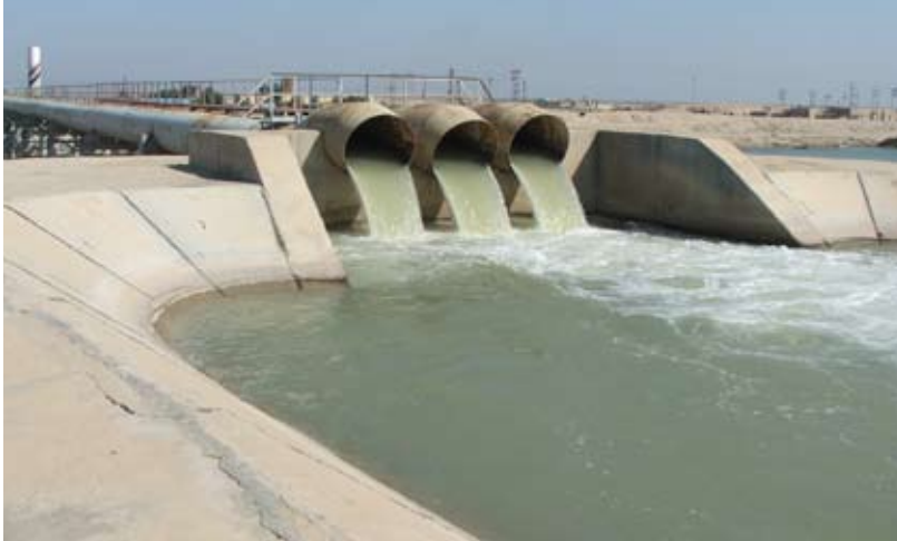
Water flowing out of all three pipelines from Pump Station #2 into the Umm Qasr Canal
