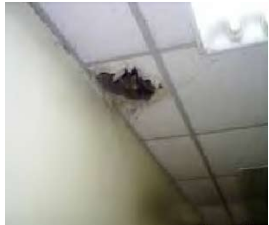
Ceiling damage caused by water leaks at teaching hospital (Phase I)
