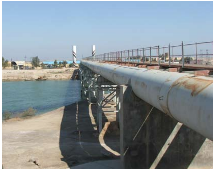
Pump Station #2, Umm Qasr Canal
