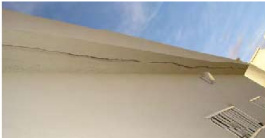
Crack in overhang of border post
