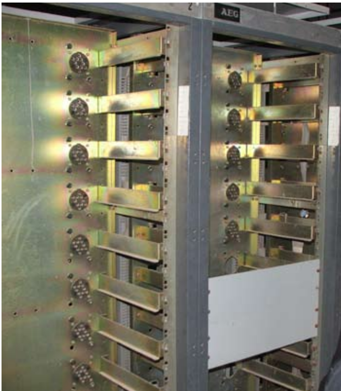
Missing electronic equipment at runway substation
