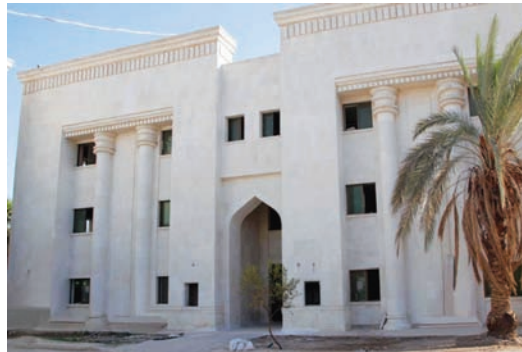
GRD is renovating a former Iraqi military headquarters site and turning it into the future Iraqi International Academy. (USACE photo)
