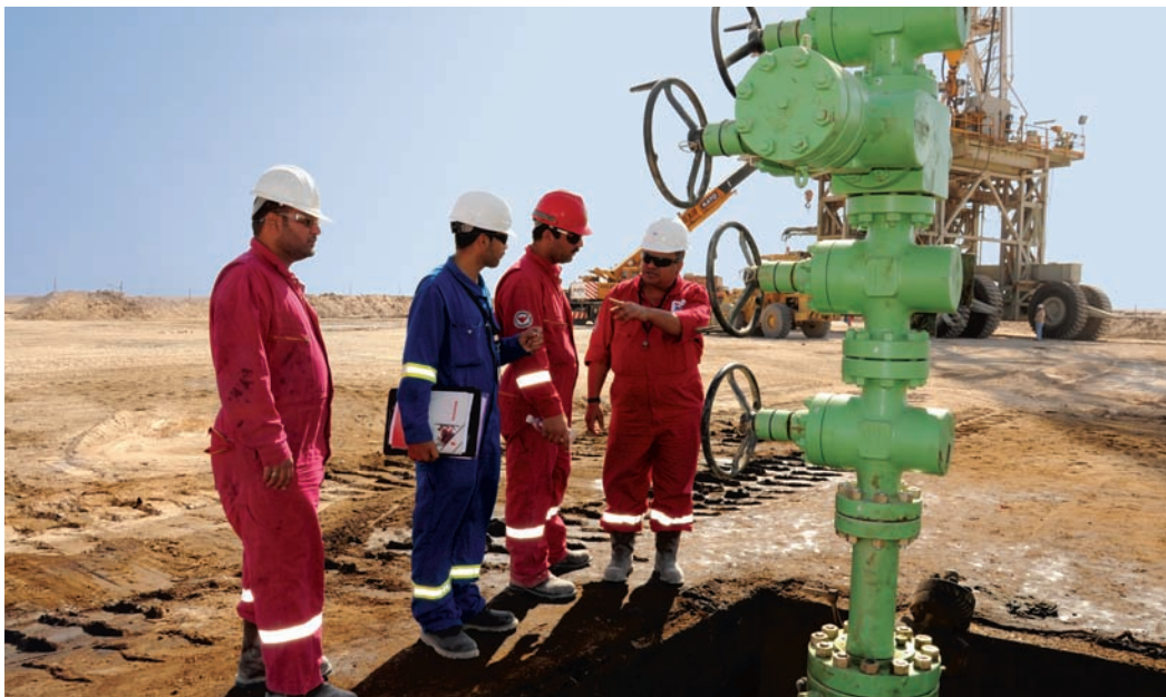
Workers at the al-Rumaila Operations Organization (ROO)—a consortium of Iraq's South Oil Company, British Petroleum, and the Chinese National Petroleum Corp.—reportedly drilled 41 new oil wells in Basrah's al-Rumaila field in 2010. Iraq's southern oil fields contain more than half of the country's proved reserves, and international oil companies are also ramping up operations at West Qurna, Majnoon, and al-Zubair. (ROO photo)
