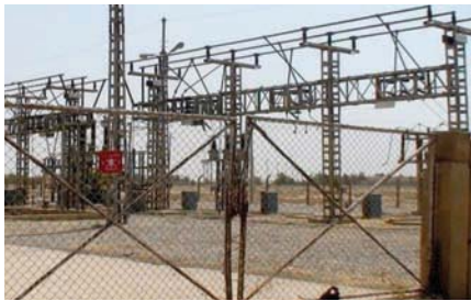
Kirkuk substation. (OPA Photo)
