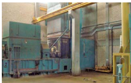
Karkh Water Treatment Plant. (USACE photo)
