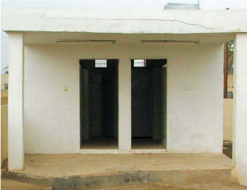
New latrine building with significant shear crack.
