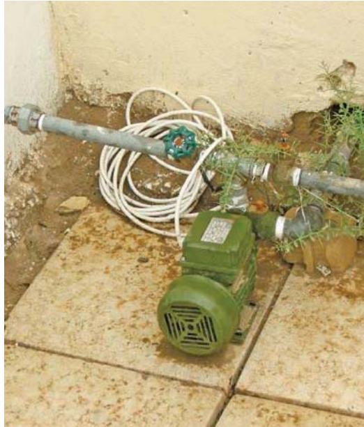
Exposed electrical wiring to the supply pump at the Khandek Intermediate School.
