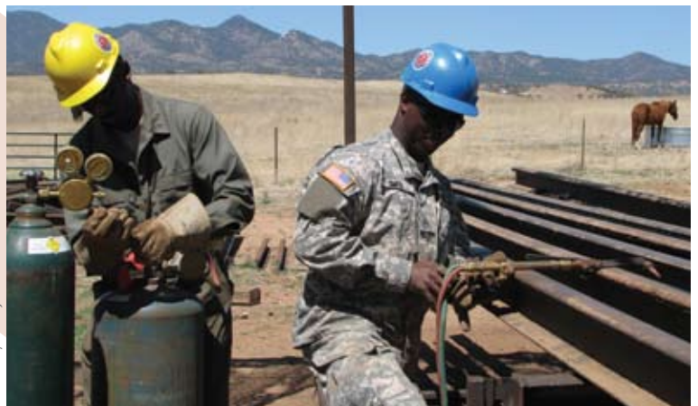
(L-R): Spc. Thomas Robinson of Anderson and Staff Sgt. Raymond Smith cut rails for vehicle barrier support beams along the U.S. – Mexico border.
