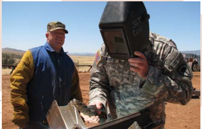
(L-R): Sgt. Jodi Cox of Landrum watches Brig. Gen. Laurie Newton of Conway spot weld a cross beam of a vehicle barrier to its support beam along the Mexican border.
