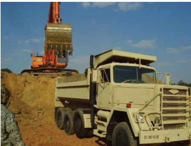
Soldiers from the 124th Engineer Company wait for trucks to be loaded so they can transport the dirt to Oak Pointe Elementary School
