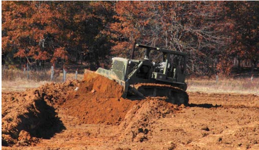
A Student operates a D7F Bulldozer during the 21E10 MOS-T Class 555-08 training. Students gain many hours of experience on four different pieces of Engineer Equipment during the two week course at the McCrady Training Center in South Carolina.
