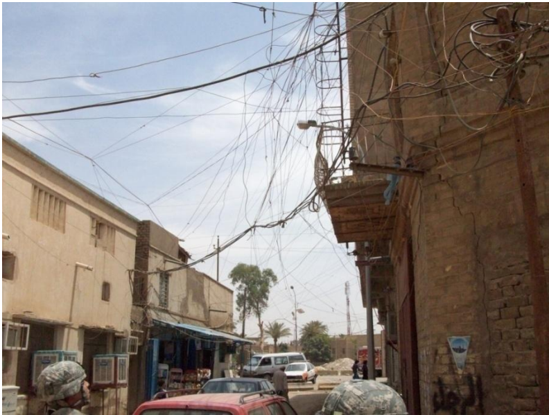
Figure 5—Resident-Installed Electrical Lines in Muhalla 312
