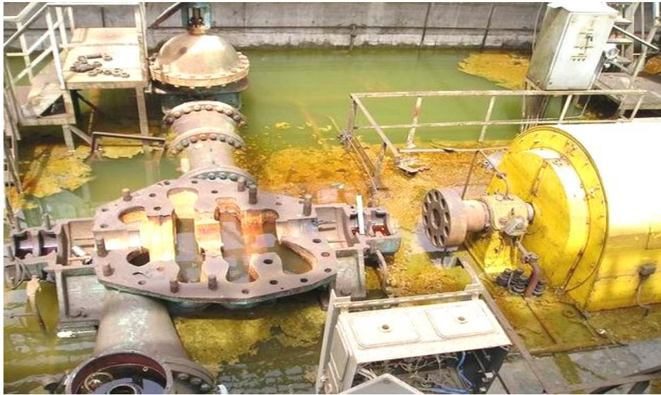
Figure 5—Ramallah Water Injection System Before Repair
