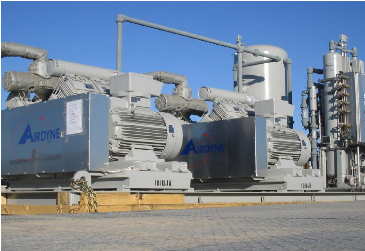
Figure 11—Task Order 20 - Compressor for Installation
