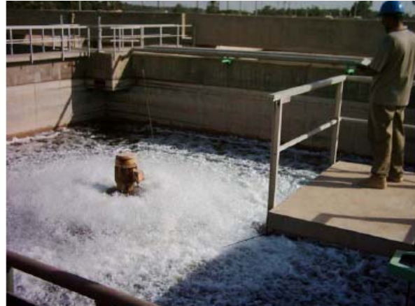
Wastewater-Treatment Plant Aerator in Operation
