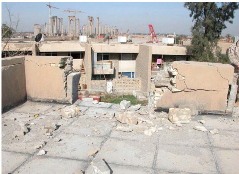
Figure 2 – Roof of Bombed Baghdad Recruiting Station
