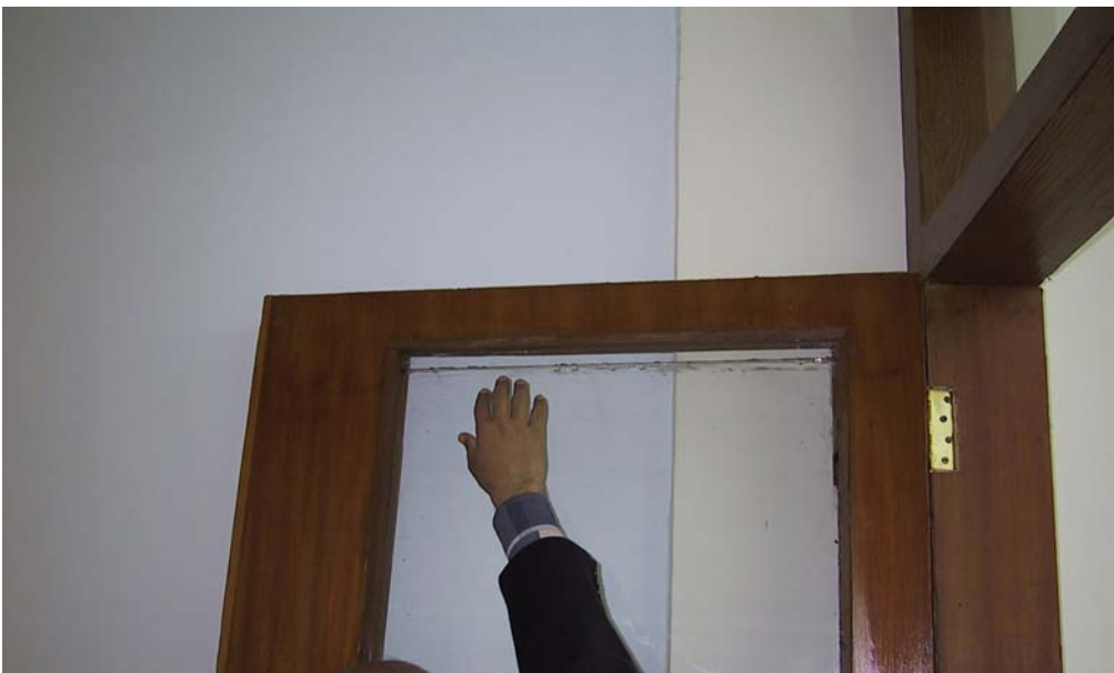
Photo 2. Improperly sized glass door panel
