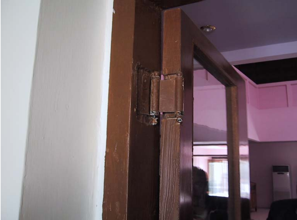
Photo 1. Incomplete door hinge repair
