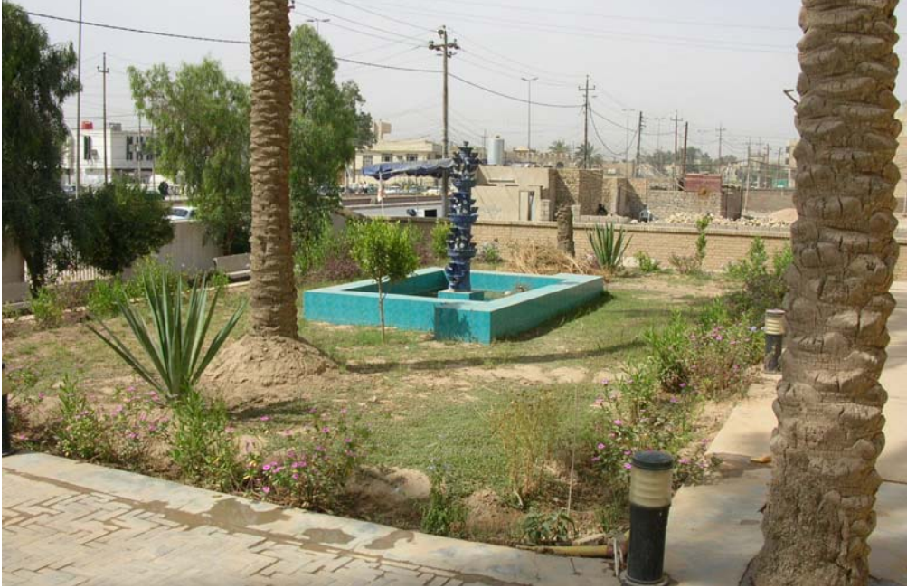
Photo 3. Inoperable fountain, missing hedge plants, and partial landscaping lights
