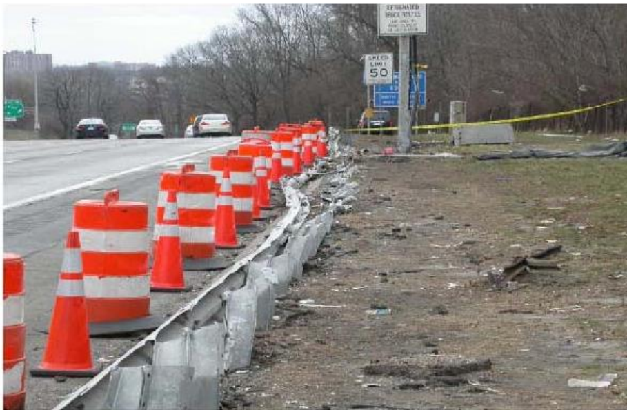
Figure 5. Damaged guardrail at the approach to the vertical highway signpost.
