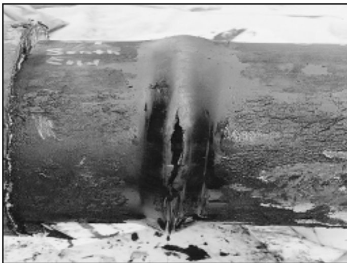
Fracture in a buckle in the pipe, Chalk Point, Maryland.
