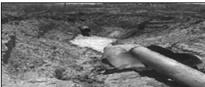
Crater created by pipe rupture, Carlsbad, New Mexico.
