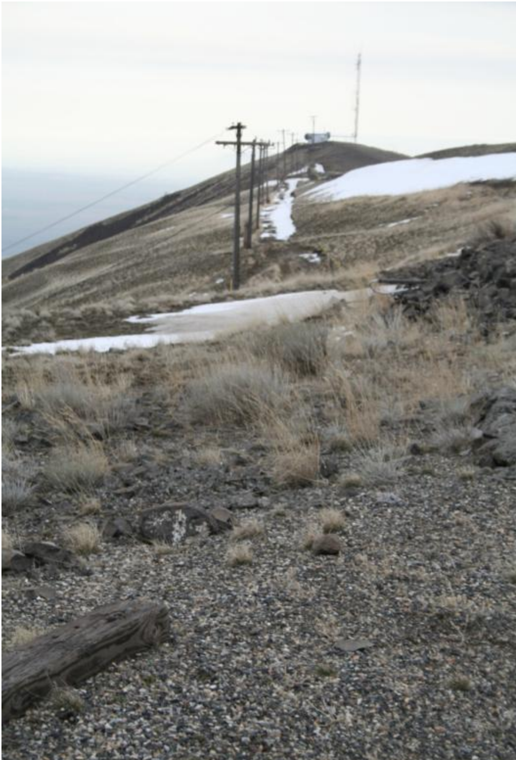
Figure A.7. Power Line (Locale 9D) to the 623-A Building (Locale 2). Photo taken at 140 degrees on 3/19/09 by Doug McFarland.
