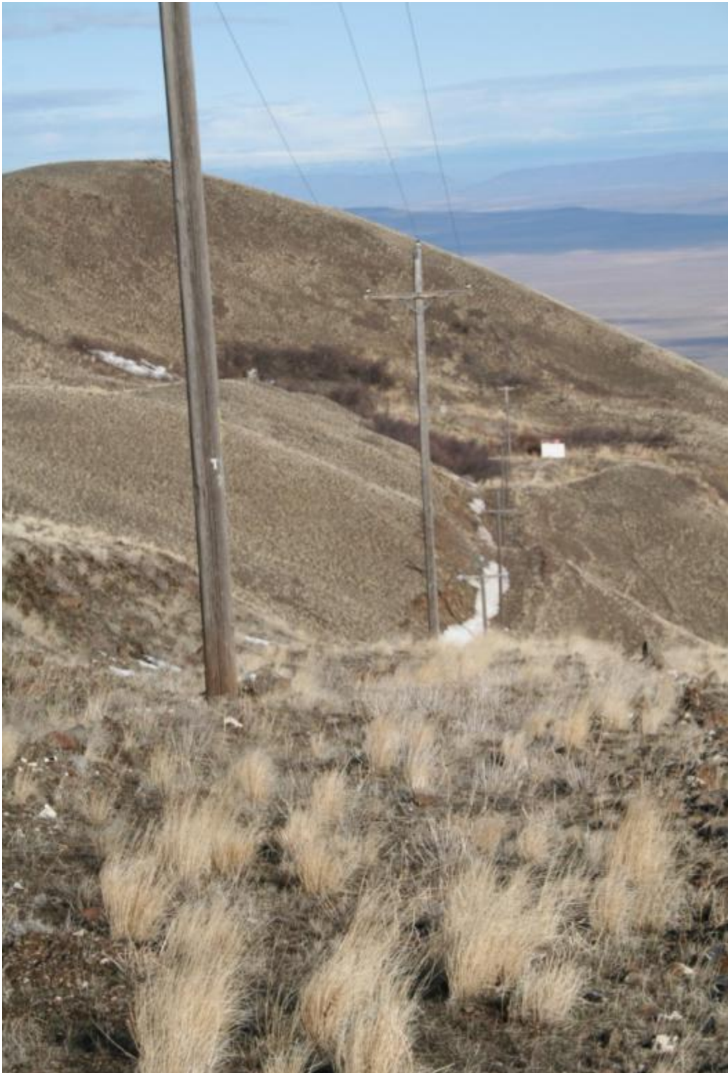
Figure A.44. Benton PUD Electrical Line (Locale 9A) and 6652-T (Locale 8) (half-way down). Photo taken at 330 degrees on 3/20/09 by Doug McFarland.
