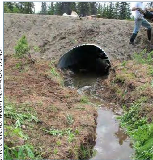
The finished culvert has a natural streambed and allows for fish passage.
