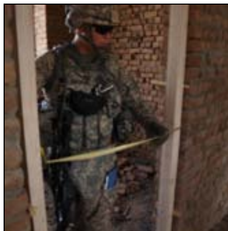
1st Lt. Jeremy Berendzen inspects an Agriculture Extension Center currently under construction in Acheen district to ensure it meets the specifications outlined in the Statement of Work. QA/QC inspections help ensure that a contractor does not "cut corners," or he risks not being paid, or even having the entire project cancelled.
