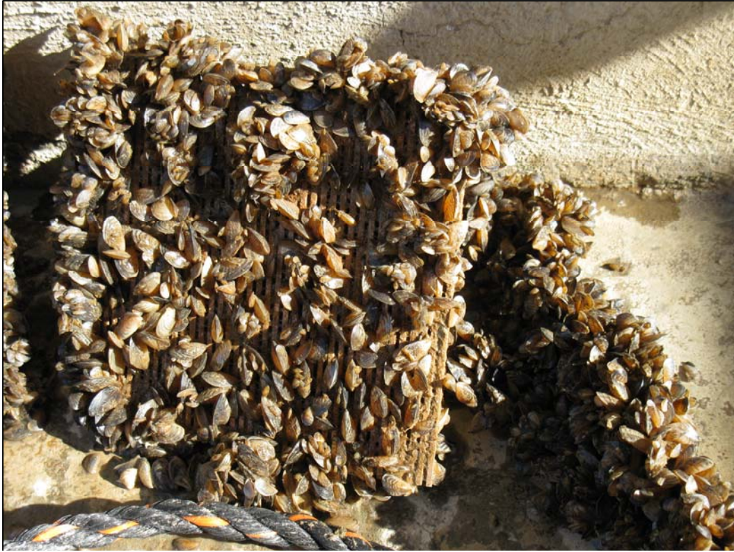
Figure B-12. This 90-10 copper nickel fish screen has been exposed for 4 months; notice the amount of mussels attached to the surface (photo courtesy of Allen Skaja, 2009).
