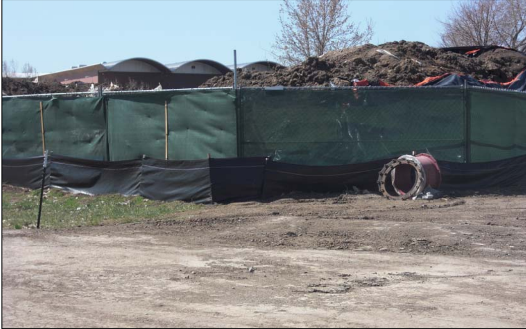
Figure A-4. Stockpiled fill material at a construction site enclosed by silt fencing to help control soil loss and the potential spread of foreign species. Black plastic covering (seen in upper right corner) has been pulled back to allow machine work (photo courtesy of Joe DiVittorio, 2010).
