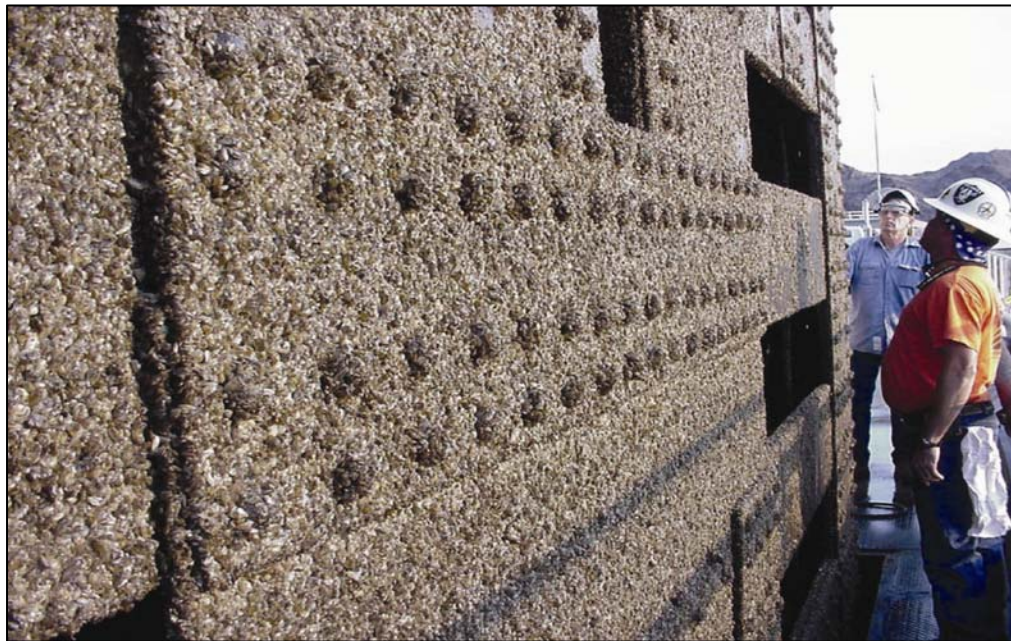
Figure A-11. Mussels covering a penstock gate at Davis Dam (photo courtesy of Dave Arend, 2008).
