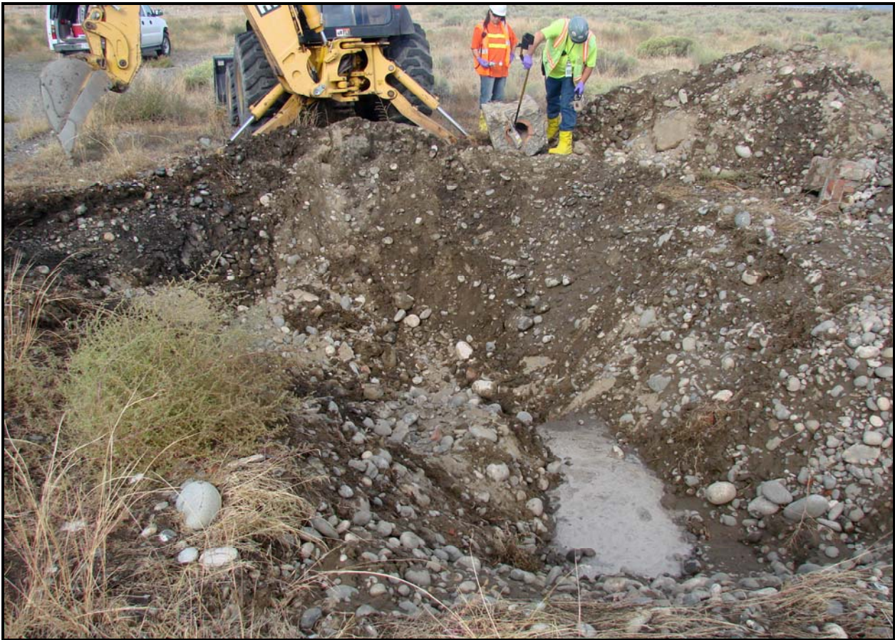
Confirmatory sampling at site 100-F-60 is complete. The site contains a pipeline. (Photo 6)
