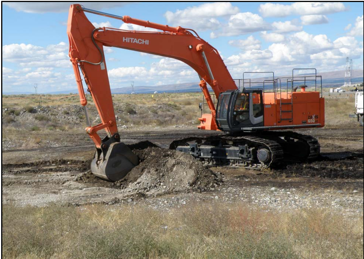
Ojeda Business Ventures works to remediate site 100-F-48. The site contains coal-pit debris. (Photo 5)
