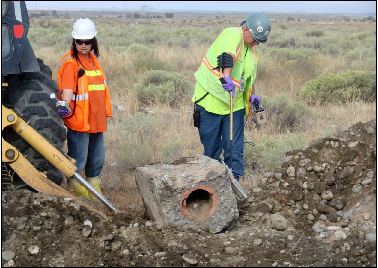
Radiological control technicians and industrial health technicians take radiological and vapor readings during confirmatory sampling of Site 100-F-60. (Photo 7)
