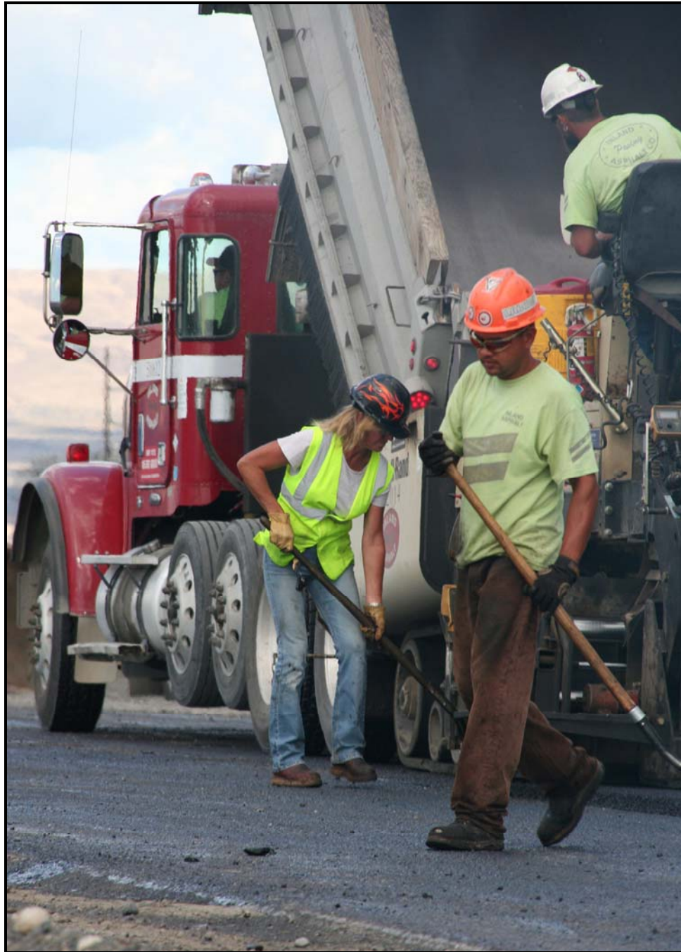
Workers from Washington Closure Hanford subcontractor Fowler General Construction pave the final section of Route 4 at the Hanford Site. (Photo 4)
